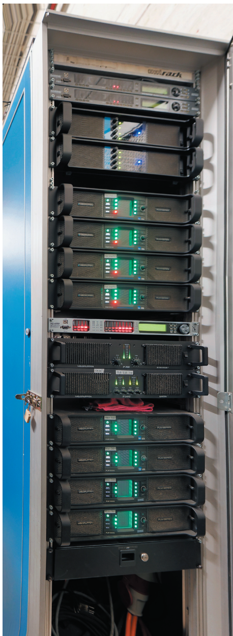
Rack cabinet with the audio electronics for the sound system in the Kulturfabrik Kofmehl. The upper group of four in the rack are the Lab.Group open amplifiers for the Stoll Convertible arrays.
